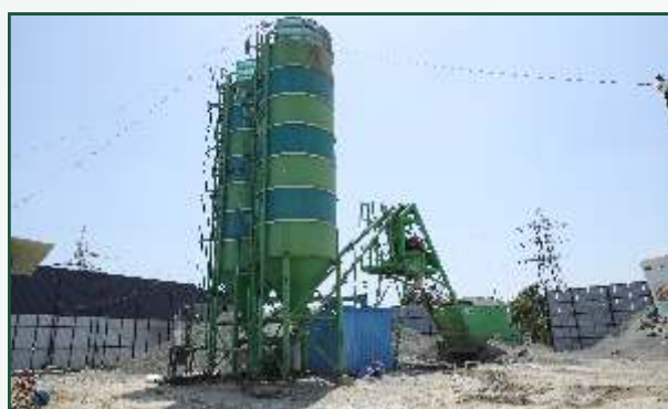
Own Concrete Manufacture Unit
